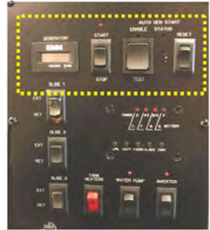
Command Center Panel
