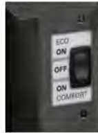
Water heater power switch
