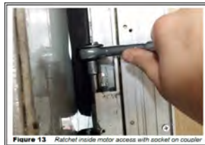
Figure 13 Ratchet inside motor access with socket on coupler
